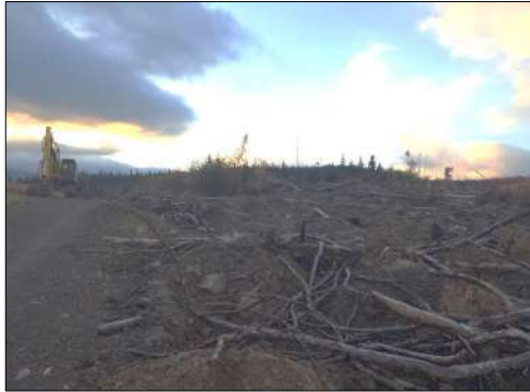
Figure 2. A site in the Callazon-Clearwater area, a recently treated road on the right, and the heavy machinery sitting on a road it is about to treat on the left.
