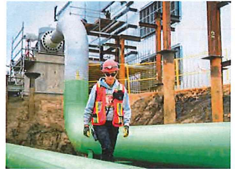
Jade began her career at Coastal GasLink as a laborer and has progressed to becoming a Civil Foreman.
